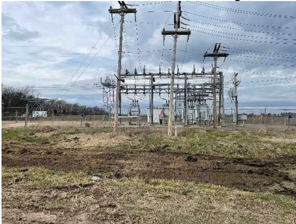
Photo 17 Electric substation on east edge of site
